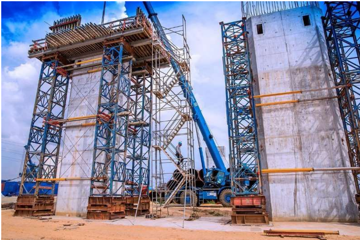
Ongoing construction of the Second Niger Bridge. The world's fastest computer costs 40 percent more than the mile-long Second Niger Bridge
